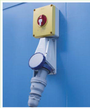
1 x 63amp IP67 plug socket for mains or generator connection
